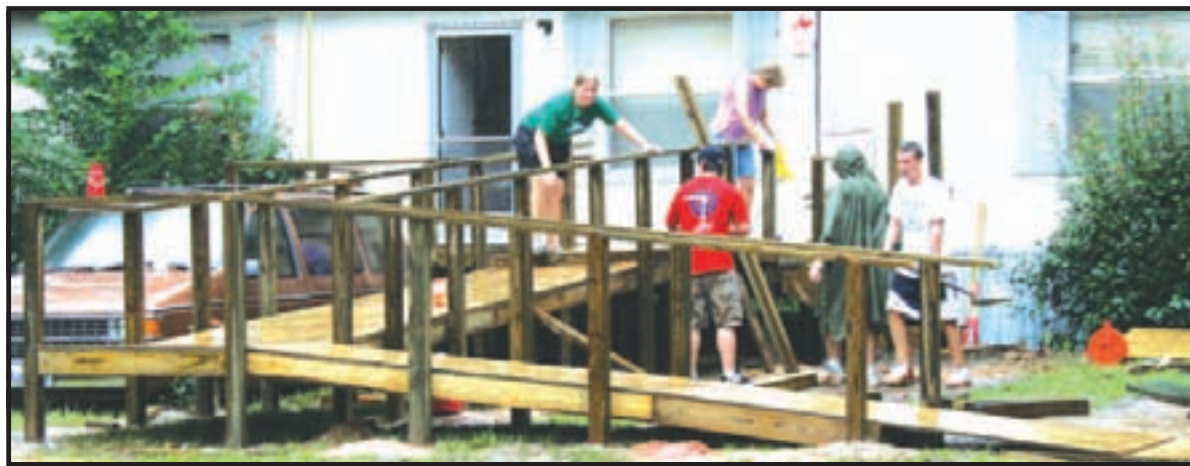
WHEELCHAIR RAMP-- A U.M. A.R.M.Y. team completes a wheel chair ramp on Big Eddy road South of Chandler during the rain last Friday. Above the team works to align the porch on Thursday.
