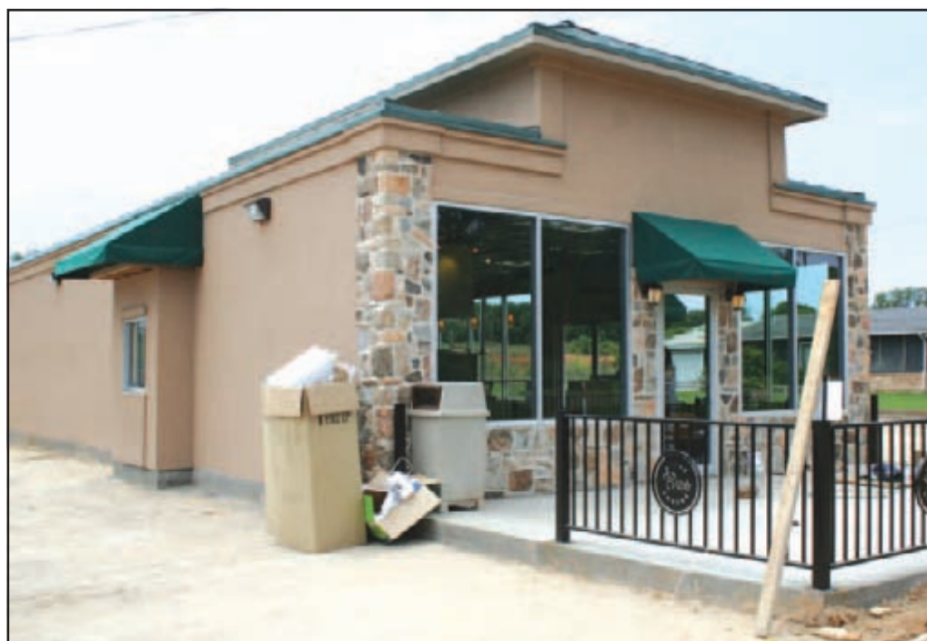
The scene on Monday as crews continued to work on Stone Brothers Coffee.
